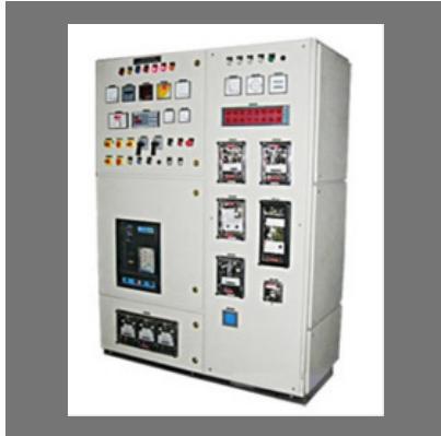
500KVA DG and Grid Protection Panel
