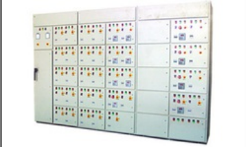
Motor Control Point Centre 40 Nos Feeder Panel
