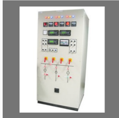
11KV TG Set with Grid SYN Panel
