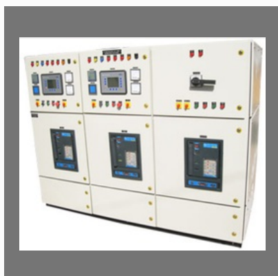
KVA DG Set with Grid SYN Panel
