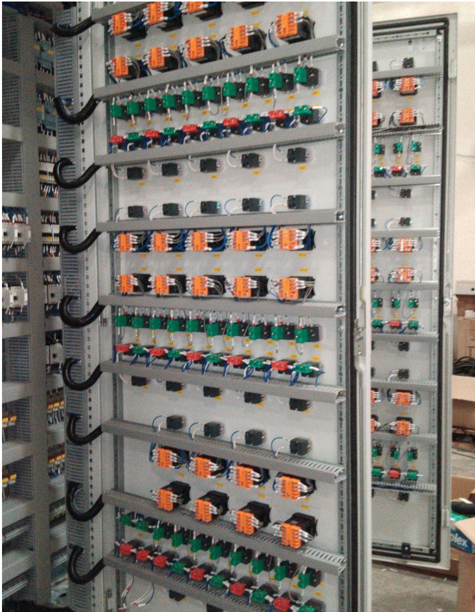
MCC Control Panel Front Door Rear Side wiring with Components
