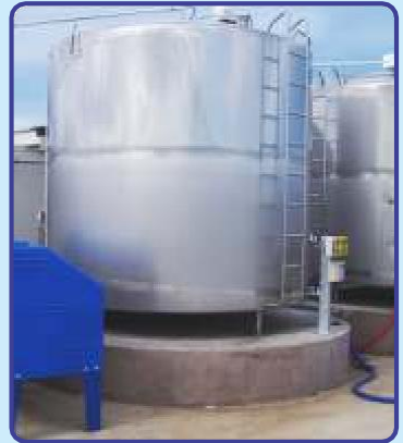
Milk Storage Tank Silo
