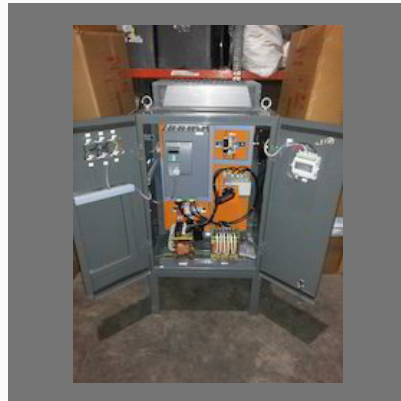
VFD Panel for Injection Moulding Machine
