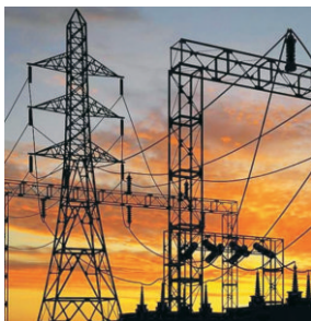
POWER GENERATION & DISTRIBUTION CENTERS
