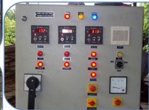
Control Panel For Automatic Operation
